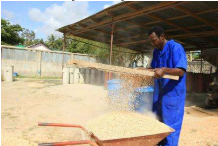
Preparing the coral stone (kokoto) before being used for building the filters (middle) & then pouring the filters (bottom)
